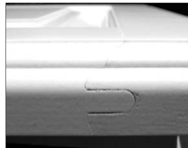
Example of end joint separation
