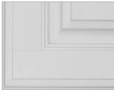
Example of front joint separation
